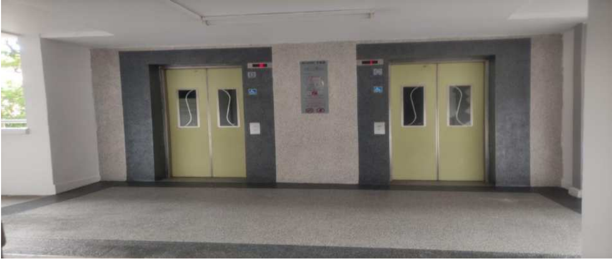
Repairs and repainting works on Lift lobby walls and floor at Blk 150 to 156 Ang Mo Kio Ave 4/5
