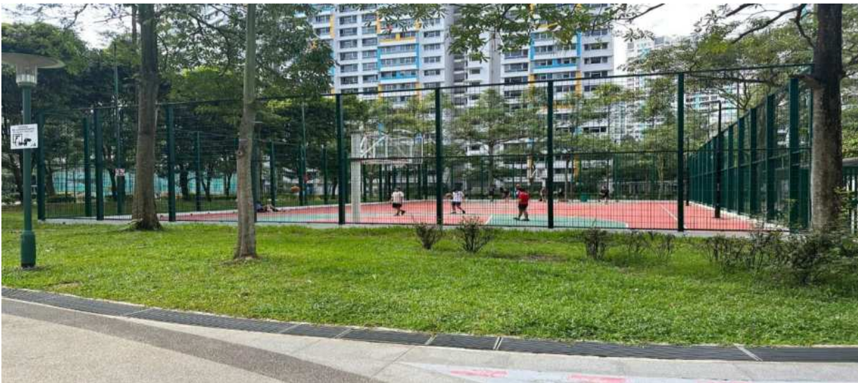
Construction of fencing to existing basketball court and installation of new floodlights at Blk 440B Fernvale Road
