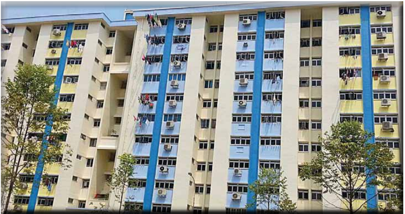
Work begins. Block 176 Ang Mo Kio Avenue 4 is the latest to benefit under the Repair and Redecorations programme.
